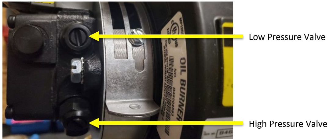
FIGURE 1-2 Burner Pressure Valves
