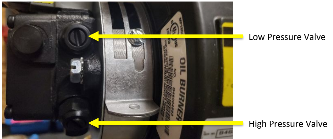
FIGURE 1-2 Burner Pressure Valves
